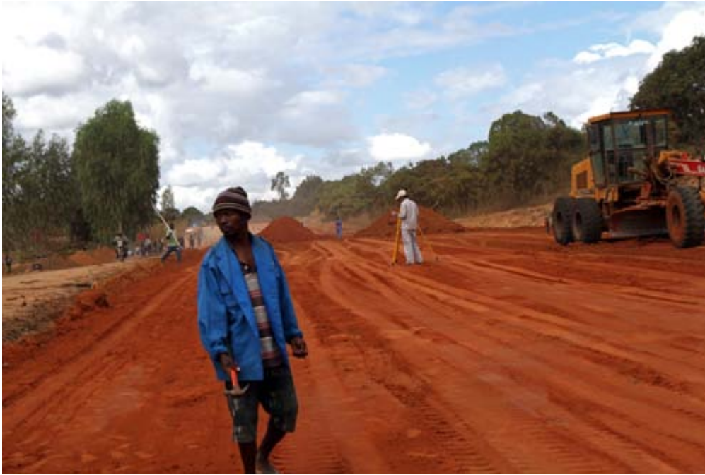
Construction of infrastructure to support large-scale agriculture is under way throughout the Nacala Corridor. (Photo: GRAIN)
