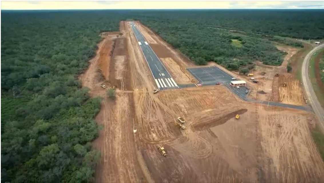
Construction of a new paved landing strip at the Infante Rivarola airfield, with access from the Transchaco Route. Credit : MOPC - Ministry of Public Works and Communications of Paraguay
