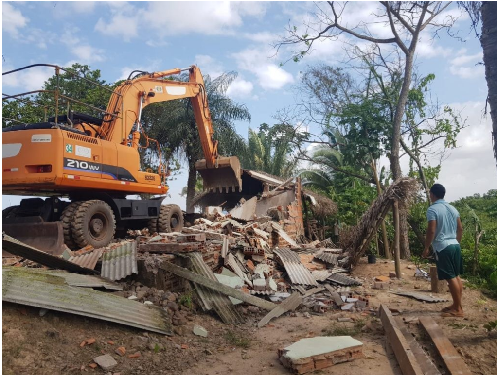
The Cajueiro (MA) community in Brazil struggling for the right to exist has its houses destroyed for the construction of the private port in the region by the WTorre construction company, in association with China Communications Construction Company (CCCC) Photo: Vias de Fato @Media Ninja
